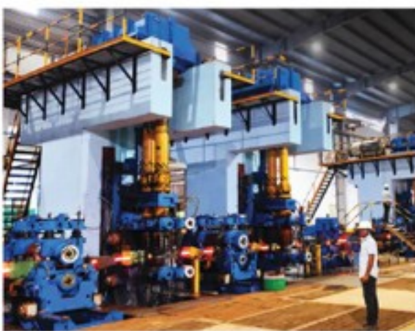
Rebar & Wire Rod Mills
